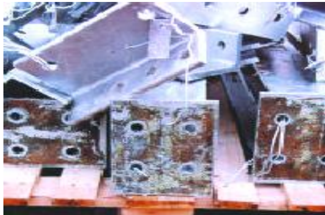
Figure20. 1. Inadequate surface preparation
