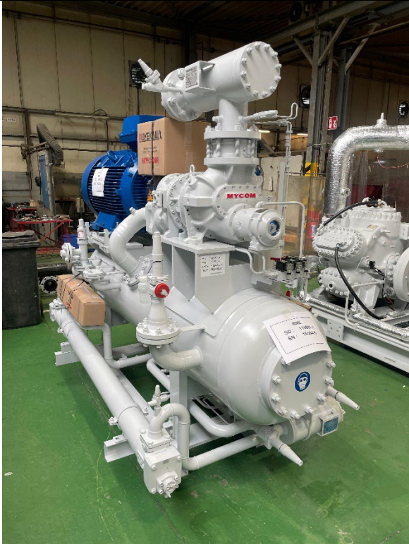
Description: Compressor Skid A (Model No. P160S / Sr. No. 1656466)
