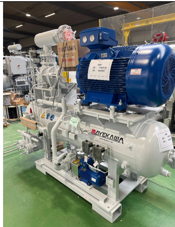
Description: Compressor Skid B (Model No. P160S / Sr. No. 1656467)
