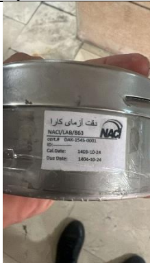
Pressure gauge calibration control
