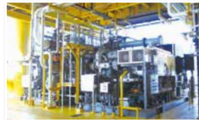
Vapor recovery compressor - Vietnam offshore 3225MMC / 600kW
