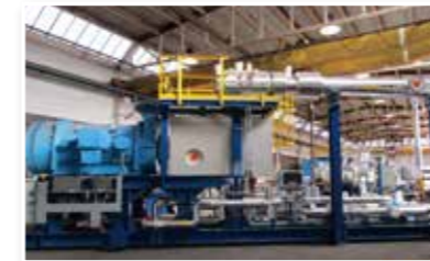
PSA compressor - Russia 400L / 1320kW
