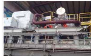
Gas chiller - Africa 4032XLLLC / 2400kW
