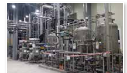
CO 2 liquefaction plant - Korea 200S / 230kW
